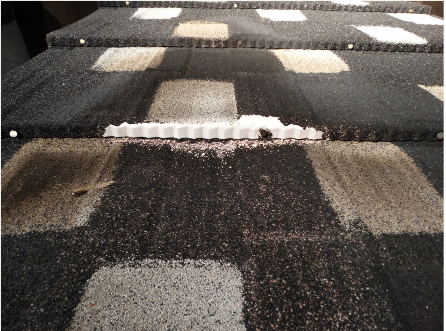
Photo 5: Spread of Flame test deck assembly after flame exposure.
